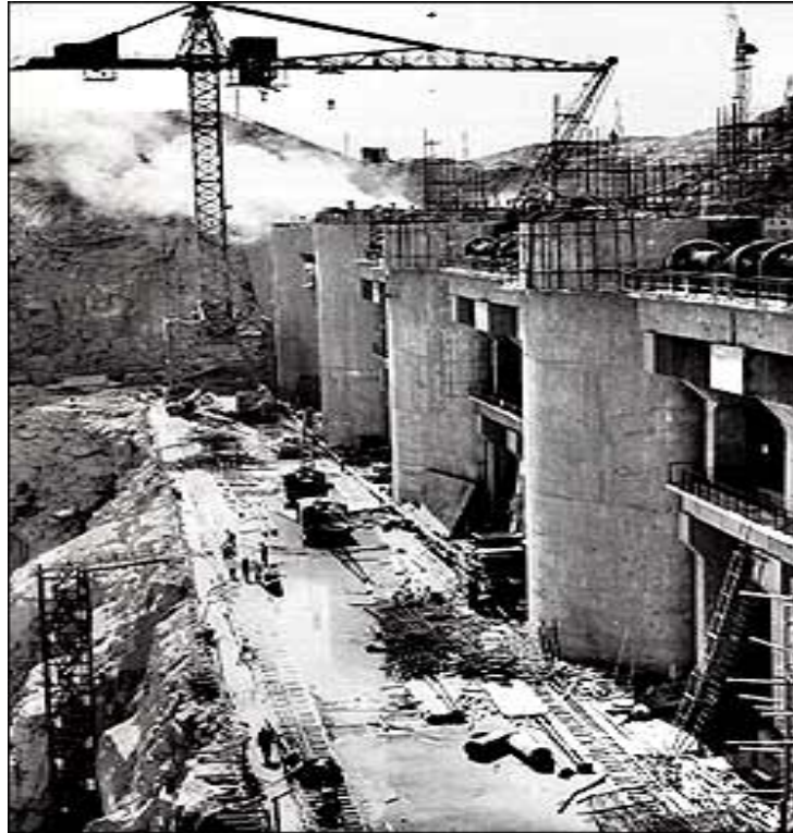
Figure 2.5: Built by Egyptian and Soviet engineers during the Nasser Era (1952-70), the Aswan High Dam is a clear example of engineering for development during the Cold War. (Source: http://www.pbs.org/wgbh/buildingbig/wonder/structure/aswam2_dam.html Credit: UPI/Corbis/Bettman. Permission Pending).
